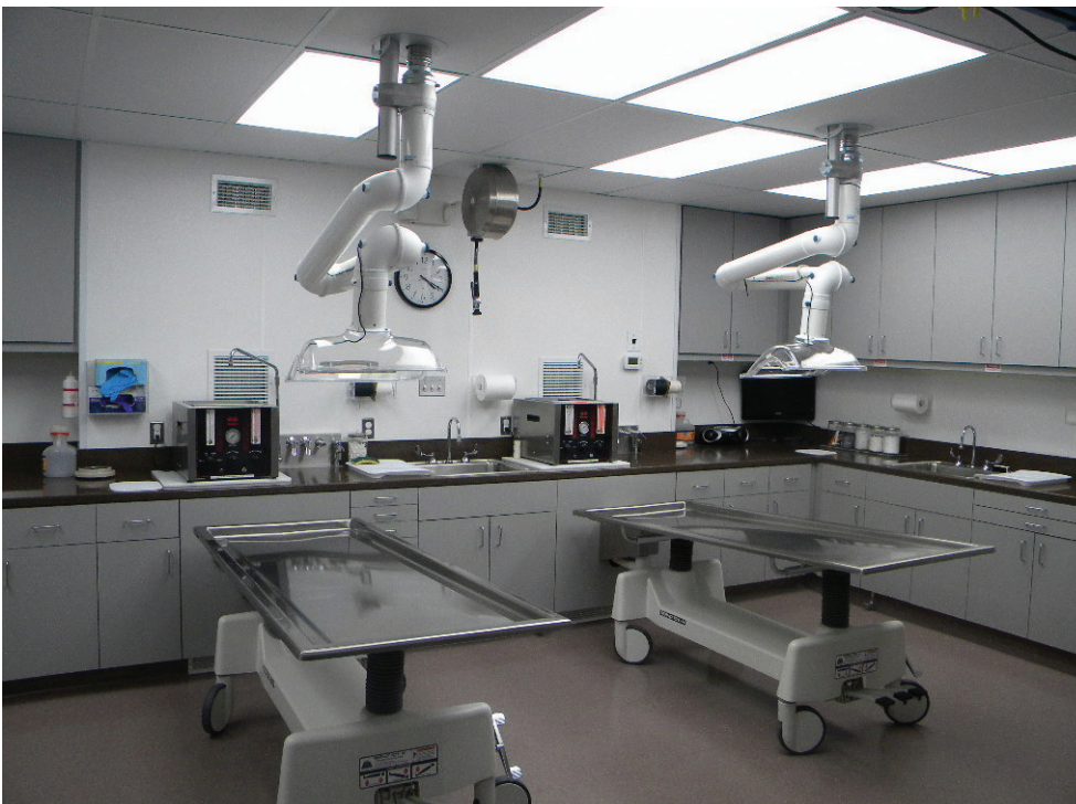
Photo: A preparation room with PrepArm, a localized air exhaust. (Photo courtesy of Duncan Stuart Todd, Ltd.)
